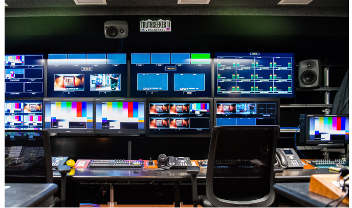
One of the control rooms at Stamford Media Center
